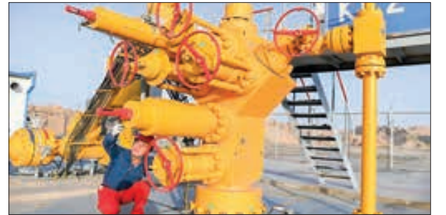
A worker checks oil transport facility at the Tarim Basin in Xinjiang Uygur autonomous region. PHOTO: XINHUA
