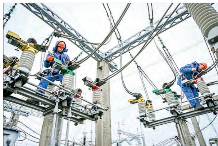
Keeping the lights on: electricians work on power lines near Balti, Moldova. PHOTO: AFP
