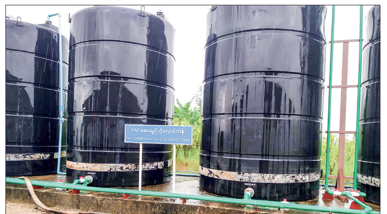
PAC Chemical Liquid Storage Tank at Ngamoeyek Water Treatment Plant (Nyaunghnapin).
