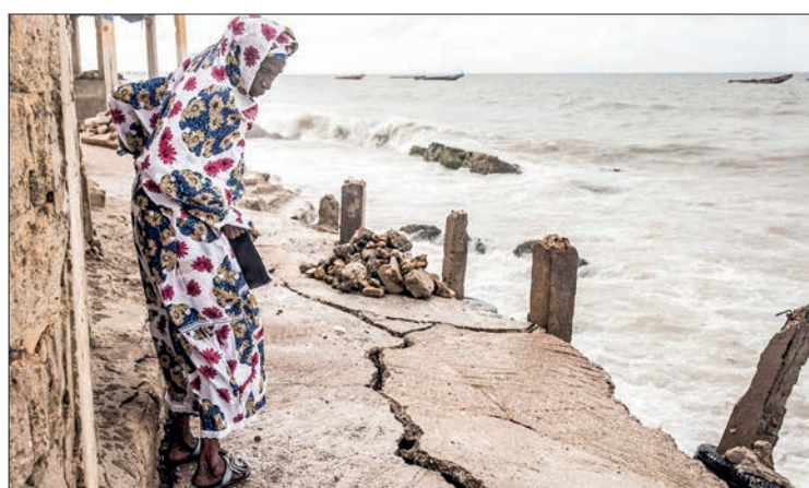
A woman looks at a newly formed crack in a walkway after a storm in Bargny, a fishing village in Senegal, on 18 Sept 2020. PHOTO: JOHN WESSELS/AFP
