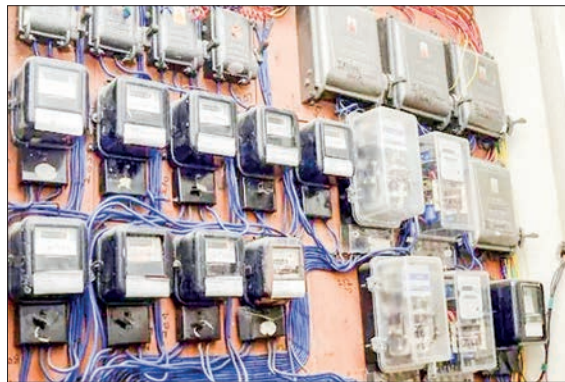
Meter boxes are seen at an apartment.
