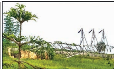
Damages of No (130) transmission Tower in the aftermath of mine attacks by PDF terrorists
