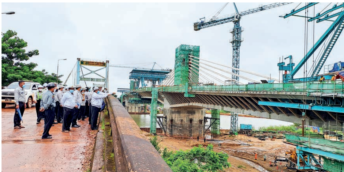
MoC Union Minister U Shwe Lay inspects the construction site of the new bridge.
