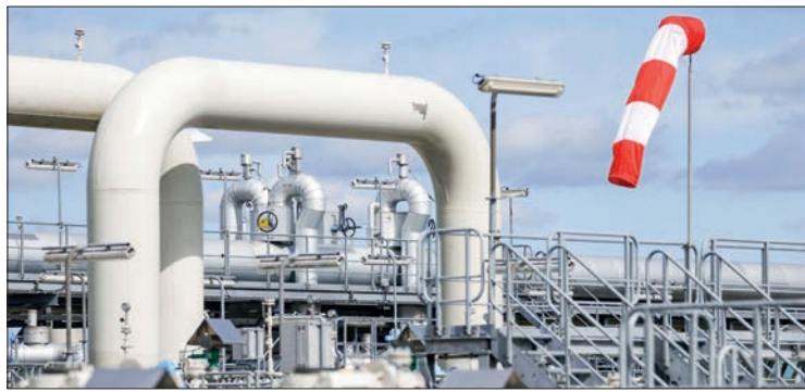
Facilities to receive and distribute natural gas are seen at a section of the Nord Stream 1 pipeline in Lubmin, northeastern Germany, on 30 August 2022. PHOTO: ODD ANDERSEN/AFP
