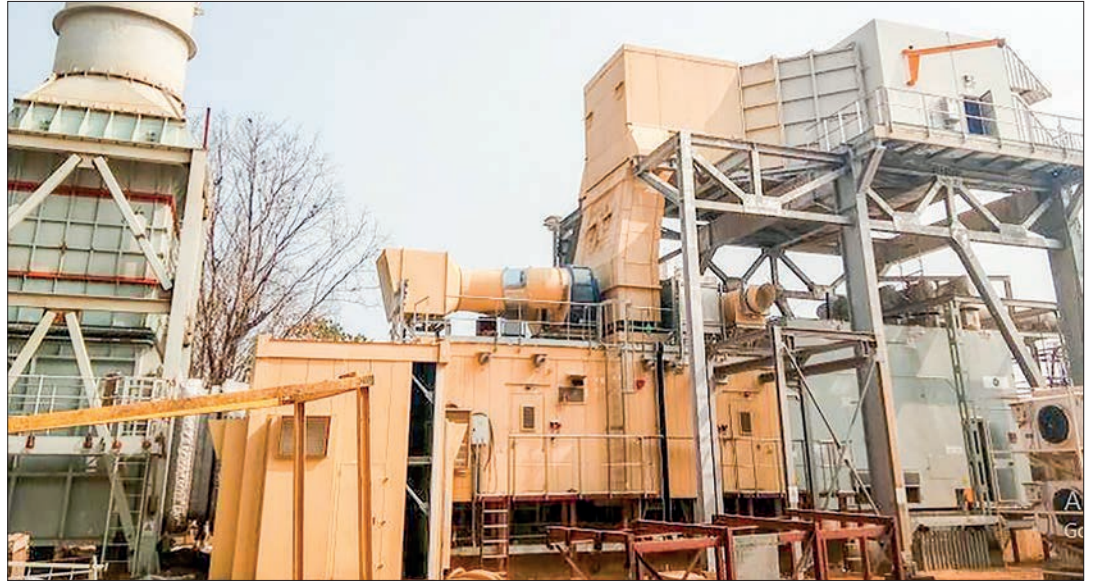
One electric power station.
