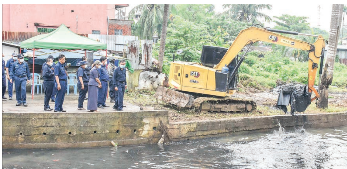
Yangon Mayor U Bo Htay and party views the drainage improvement works yesterday.
