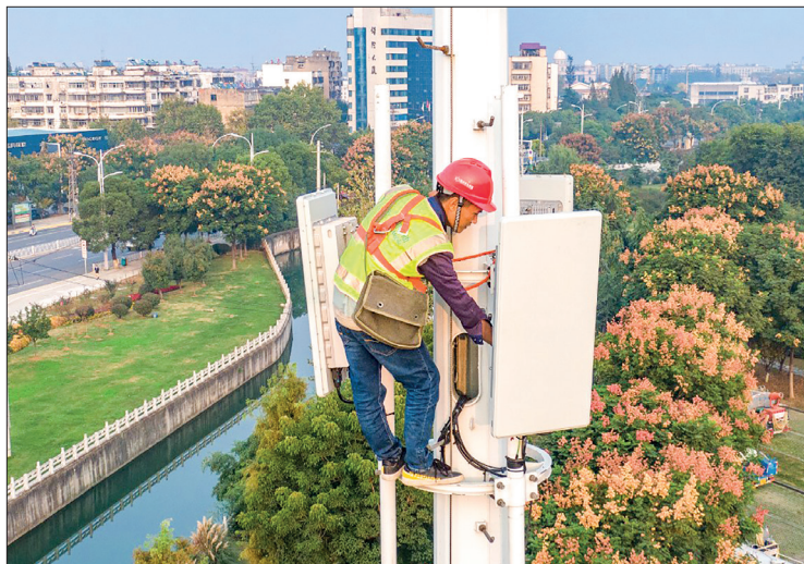
File photo of a technician on a 5G telecom tower. PHOTO: AFP
