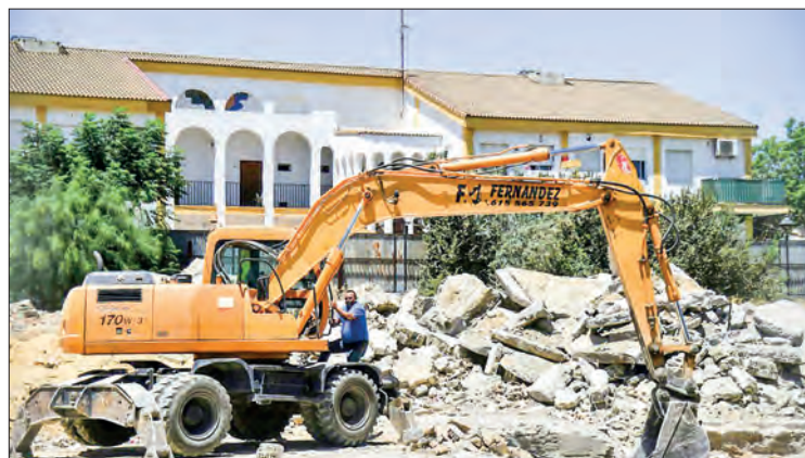
Outdoor workers, such as this demolition site worker in Seville, face health threats from extreme heat. PHOTO: CRISTINA QUICLER/AFP
