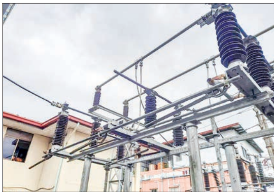
One power distribution station.
