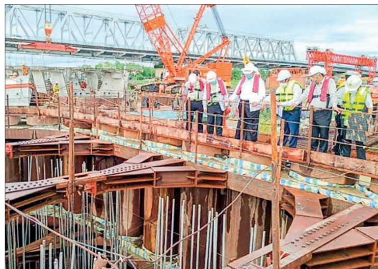
Union Minister for Construction U Shwe Lay inspects progress of Thanlyin Bridge No. 3 on 2 July.
