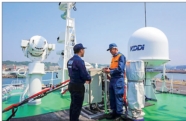
Coast Guard members inspect KDDI's cellphone base station equipment installed on their patrol vessel on 23 May 2014 in Shibushi, Kagoshima, Japan. PHOTO: KDDI/KYODO/FILE
