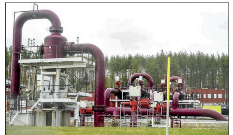
A photo taken on 12 May 2022 shows pipes at the Gasum plant in Raikkola, Imatra, Finland. PHOTO: VESA MOILANEN /AFP
