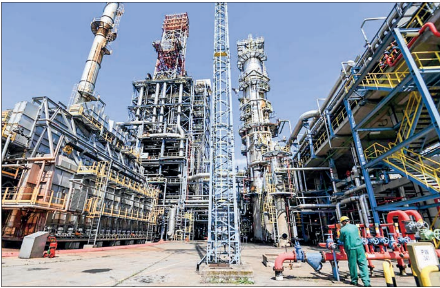
Processing and refining structures stand at the Duna oil refinery operated by MOL Hungarian Oil and Gas Plc in Szazhalombatta, Hungary, The Duna Oil Refinery still receives Russian crude. PHOTO: ATTILA KISBENEDEK/AFP
