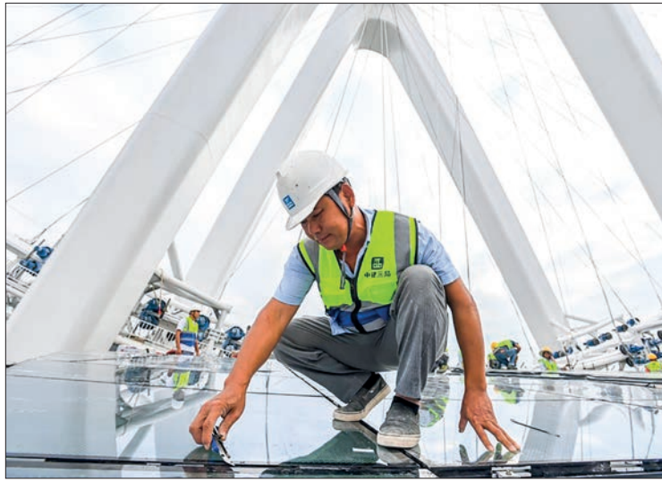
A staff member works at the construction site of a ferris wheel at Baoan coastal cultural park in Shenzhen, south China's Guangdong Province, on 6 Oct 2020. PHOTO: XINHUA/LIU DAWEI
