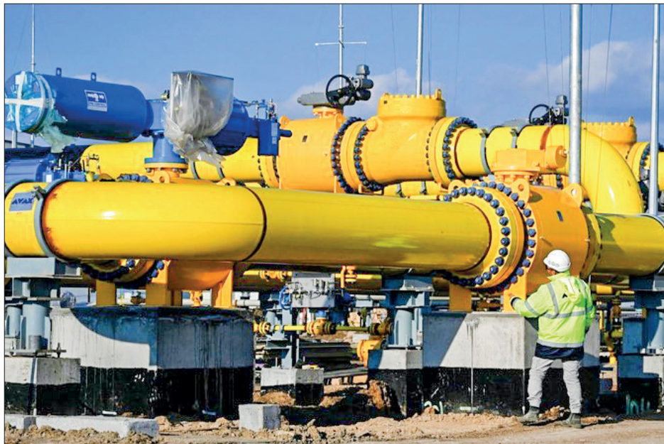
An employee checks a pipe at the construction site of a gas metering station, part of the pipeline link between Bulgaria and Greece. PHOTO: AFP
