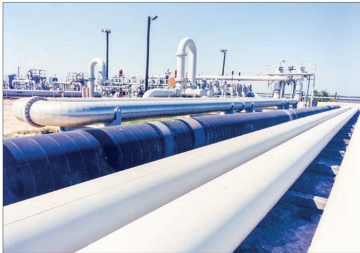
An undated photo provided by the Department of Energy shows crude oil pipes at the Bryan Mound site near Freeport, Texas. PHOTO: DEPARTMENT OF ENERGY/FILE
