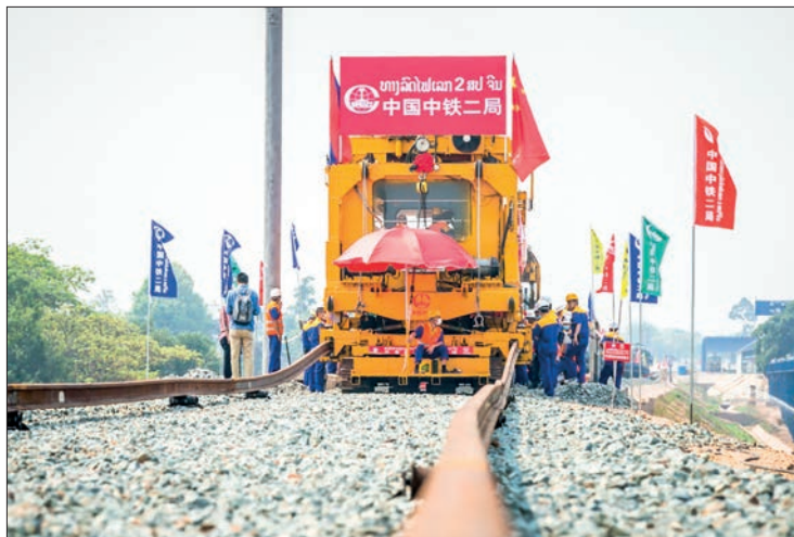
Workers lay tracks at the construction site of the China-Laos railway in Vientiane, Laos, 27 March 2020. PHOTO: KAIKEO SAIYASANE/XINHUA/FILE
