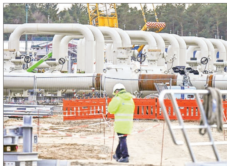
A worker at the construction site of the Nord Stream 2 gas pipeline in Lubmin, northeastern Germany. PHOTO: AFP / TOBIAS SCHWARZ
