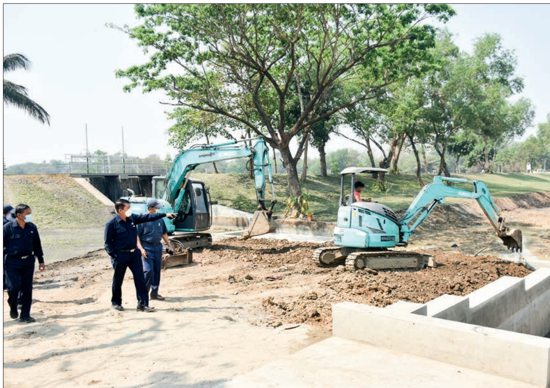
Yangon Mayor U Bo Htay views dredging of waste and sand at No 1 drainage outlet in Shwelinban Industrial Zone in Hlinethaya Township on 27 February.
