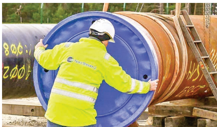
In this file photo taken on 26 March 2019 a worker puts a lid on a pipe at the construction site of the Nord Stream 2 gas pipeline in Lubmin, northeastern Germany. PHOTO: AFP
