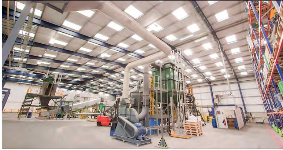
Located within 2 hours west of London, BASF's state-of-the-art recycling facility at Cinderford in Gloucester, UK is fully dedicated to the recovery of precious metals from spent automotive catalytic converters. PHOTO: BASF/XINHUA
