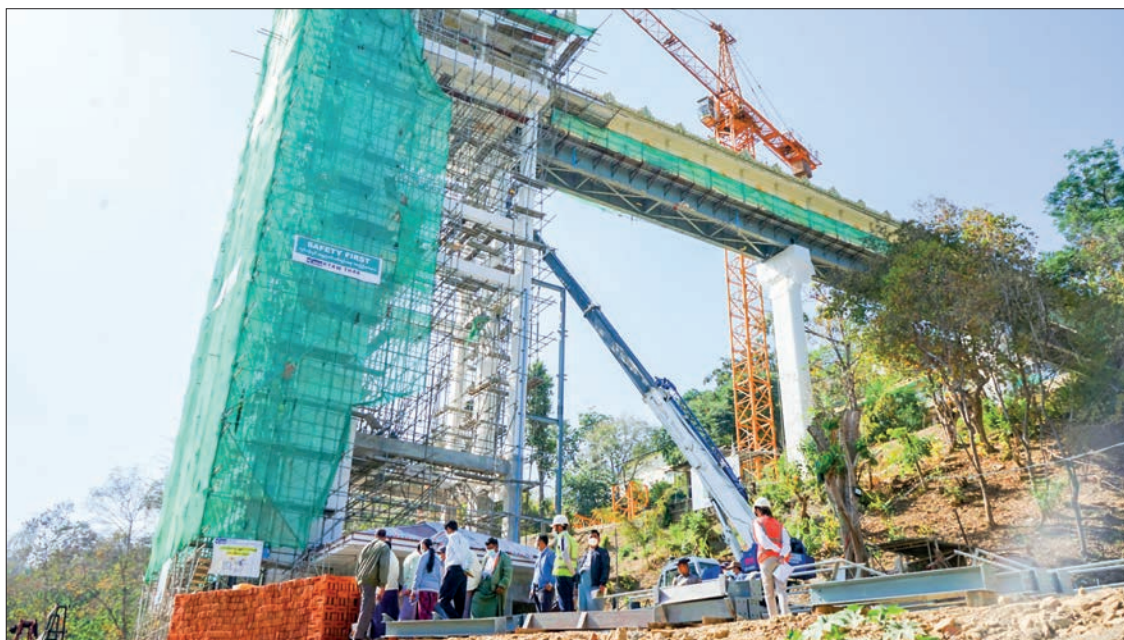
A lift tower is under construction at Mann Shwesettaw Pagoda in Minbu Township with the use of heavy machinery.
