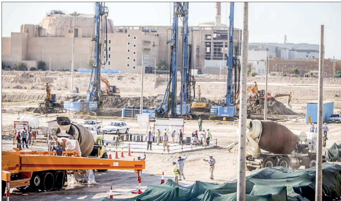
Laborers work at the construction site of the second phase of Iran's Bushehr Nuclear Power Plant in Bushehr, southern Iran, on Nov. 10, 2019. PHOTO: AHMAD HALABISAZ/XINHUA
