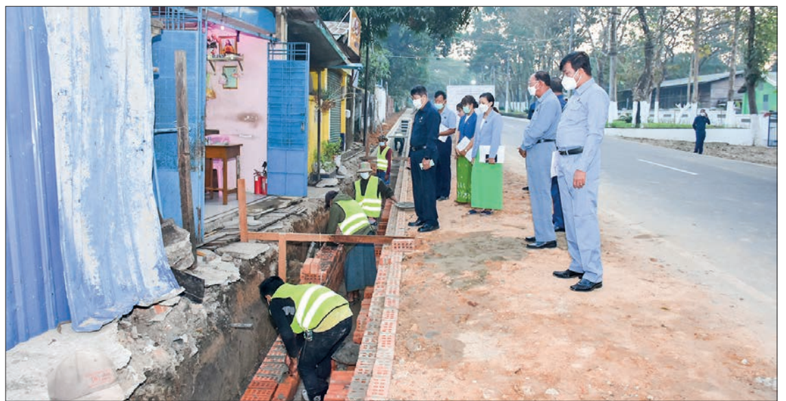
Yangon Region Minister for Development Affairs U Bo Htay views construction of drains in Thanlyin Township on 23 January.
