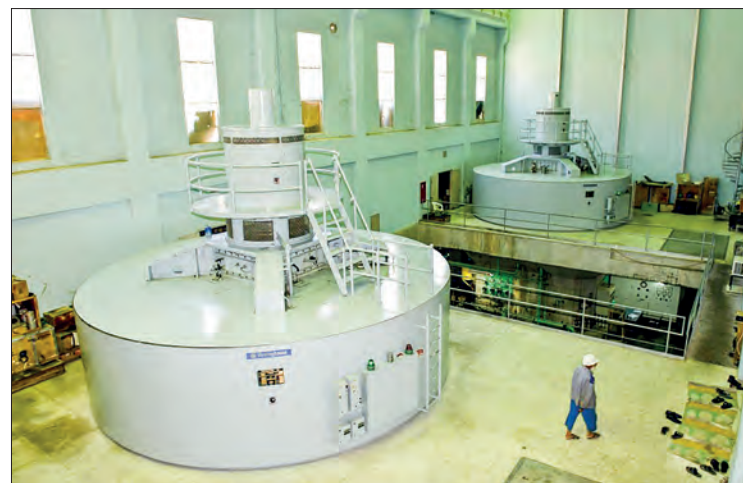
Inside the power station at the Kajaki Dam in the southern Helmand Province of Afghanistan. PHOTO: WIKIWAND/ANI
