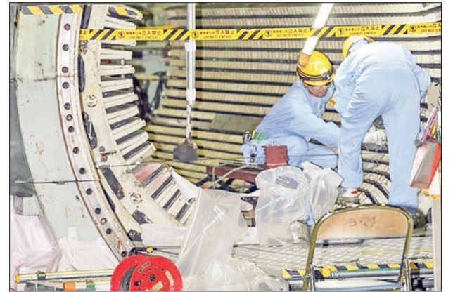
Workers dismantle the Unit 2 reactor at Chubu Electric Power Co.'s Hamaoka nuclear power plant in Omaezaki, Shizuoka prefecture. PHOTO: KYODO / FILE
