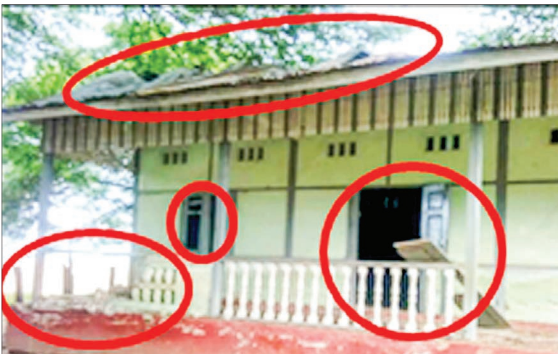
School building seen hit by handmade mines in Singu Township, Mandalay Region.
