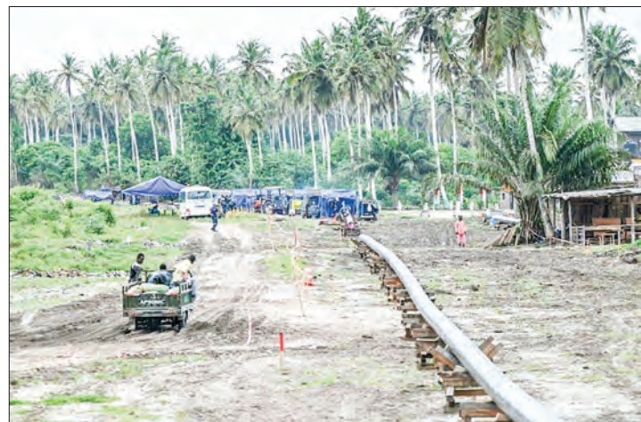
Pipelines are being laid to bring the offshore gas to power stations under construction in Abidjan and Jacqueline. PHOTO: AFP
