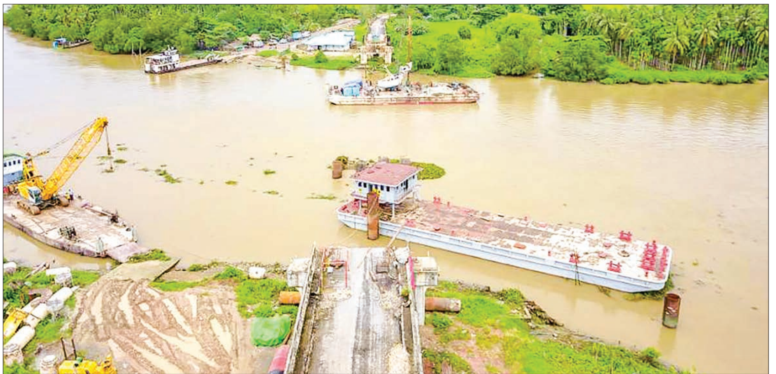
The upgrade works started on 2 October 2020 and are estimated to complete in the 2022-2023 financial year, according to the ministry.
