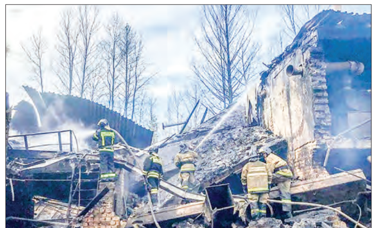
Russia's emergencies ministry said the fire could have broken out as a result of "violations of technological processes and safety measures". PHOTO: RUSSIAN EMERGENCY SITUATIONS MINISTRY/AFP
