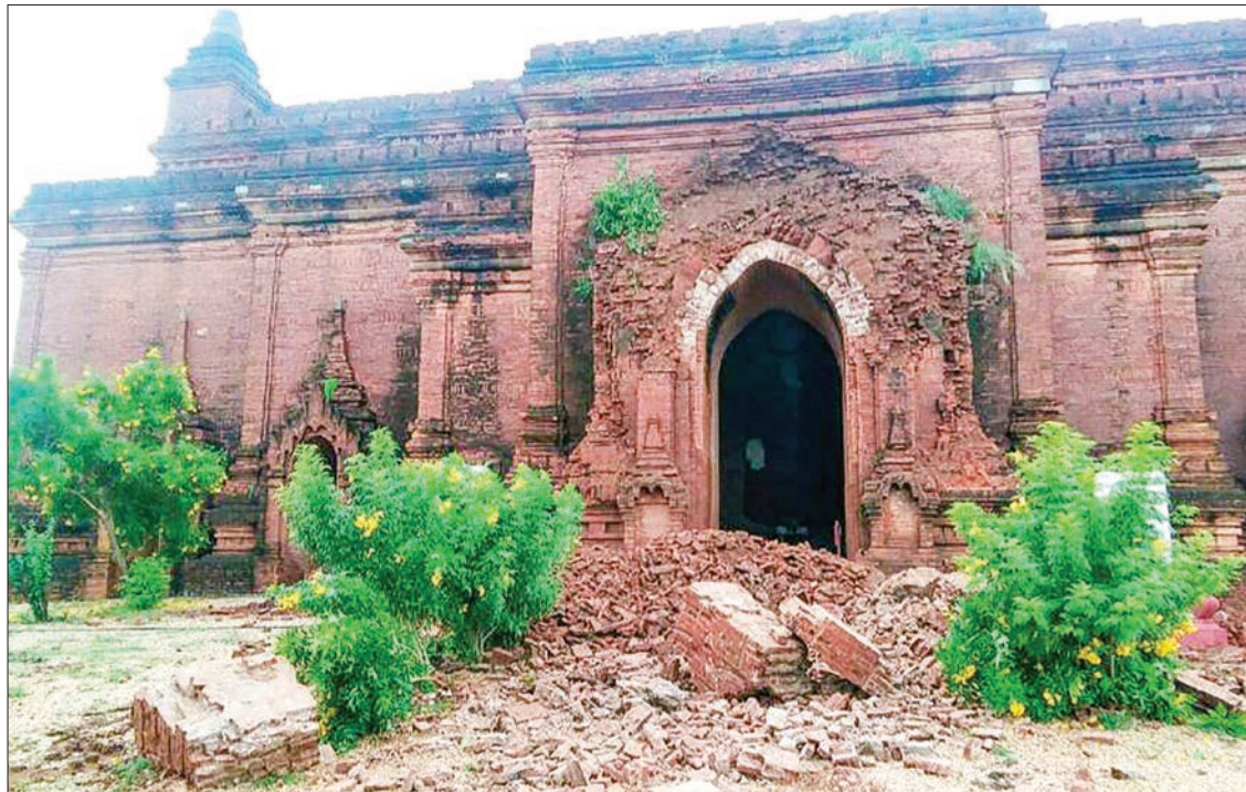
Some damages are seen in the aftermath of the torrential rainfall on 17-18 October in Bagan NyaungU.
