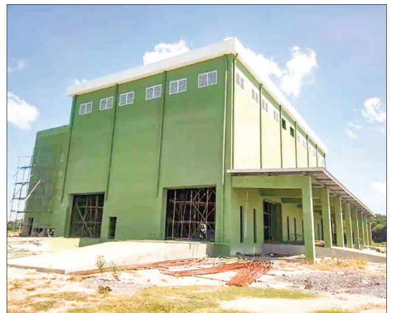
The Shwebo seed processing plant seen complete and ready to operate in December.
