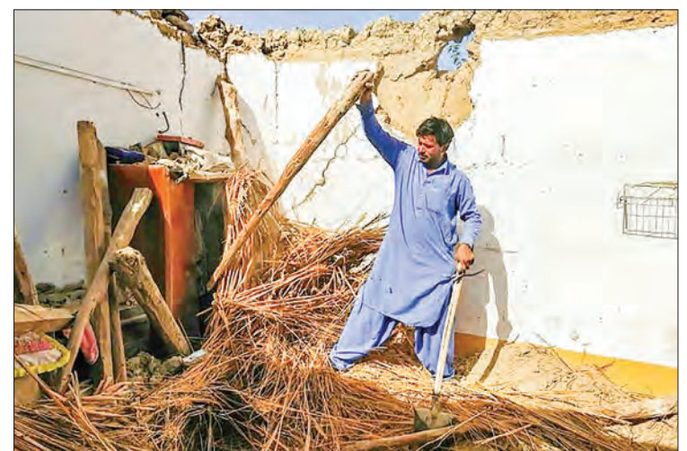
Many of the victims died when the roofs and walls of their mud houses collapsed after the 5.7 magnitude quake struck in darkness. PHOTO: AFP
