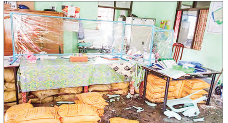
Mayangon administration body office is damaged by handmade bomb.
