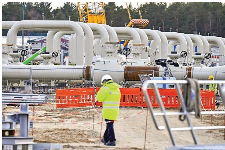
A worker walks at the construction site of the Nord Stream 2 gas pipeline in Lubmin, northeastern Germany. PHOTO: AFP / TOBIAS SCHWARZ.
