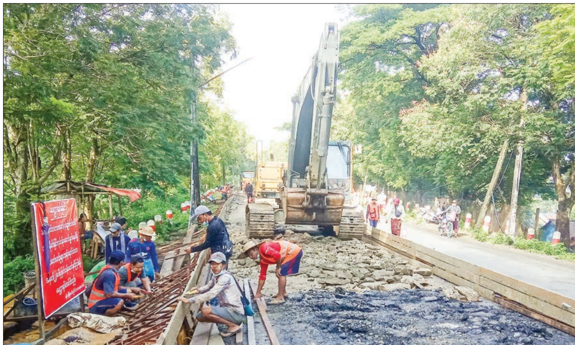
Double-layer paving of concrete approach road to Bayintnaung Bridge-1 is stepped up.
