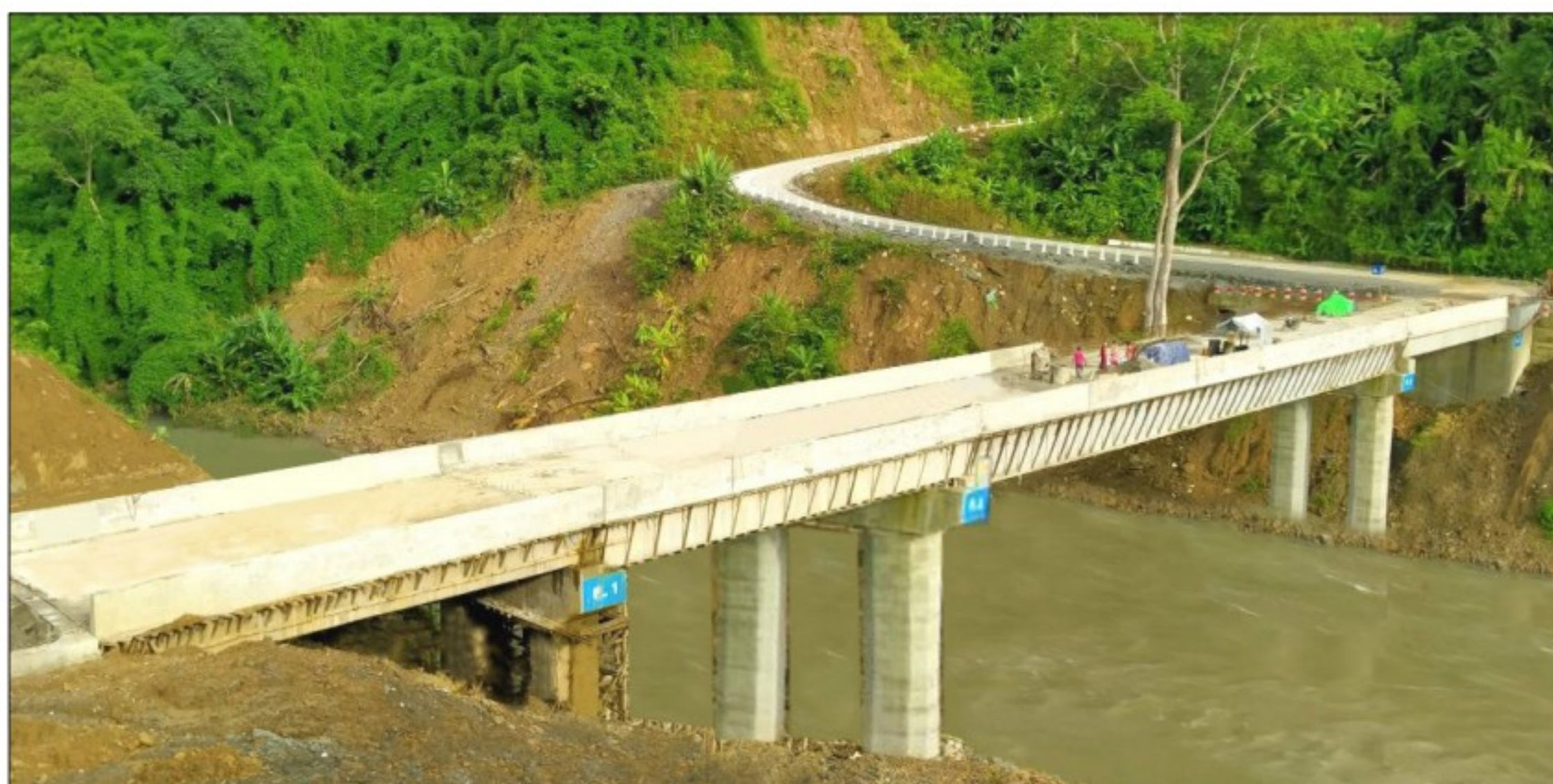
A view of the new Nantsalein creek Bridge will be built soon in Hkamti Township, Sagaing Region.
