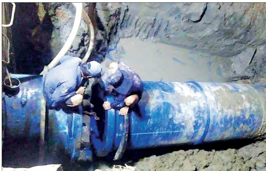
Skilled workers are connecting water pipelines for supply of water being implemented by YCDC.
