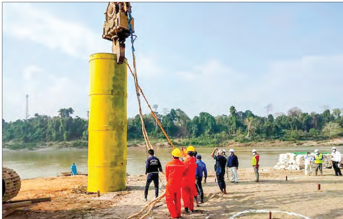
The project was launched with K2 billion of the Union budget in the 2020-21 financial year. And the Bridge Department's Construction Team (2) is taking responsibility for building Chindwin Bridge (Htamanthi) project in Homalin Township.
