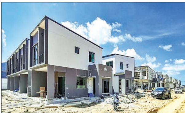
Photo shows townhouses under construction as part of the Thepharak project in Samut Prakan Province in Thailand. PHOTO: HANKYU HANSHIN PROPERTIES CORP./ NNA/KYODO
