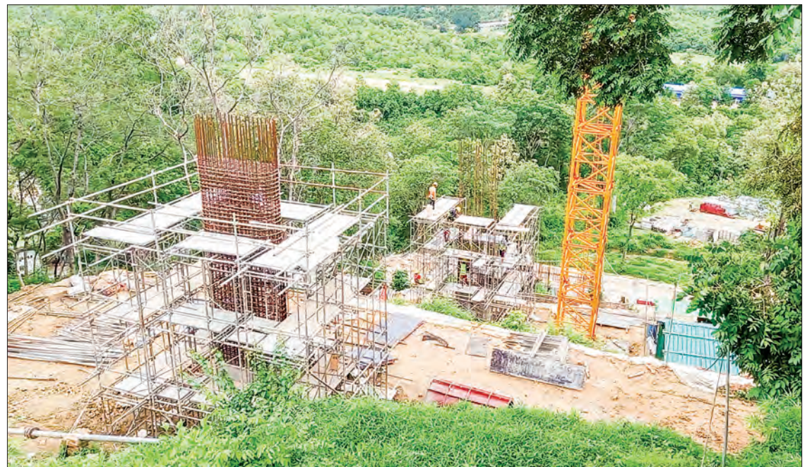
The construction site for elevator at Mann Shwesettaw Pagoda is in progress.
