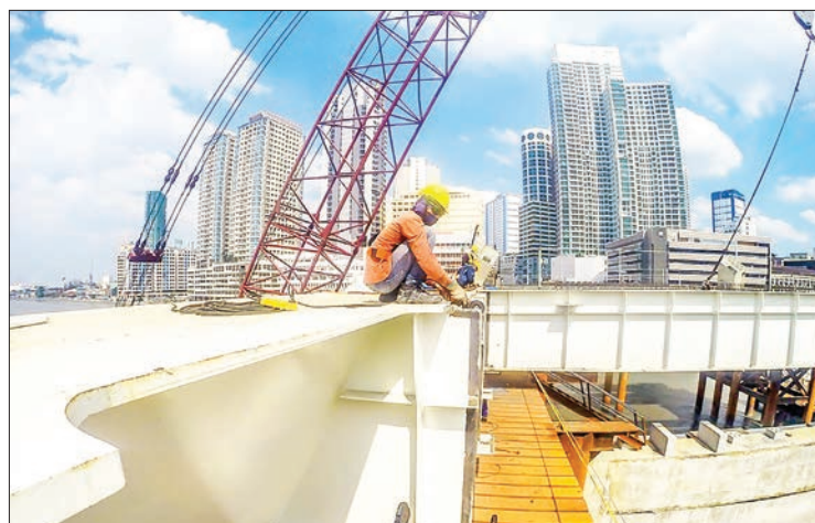
Workers work at the construction site of the China-funded Binondo-Intramuros Bridge in Manila, the Philippines, Nov. 18, 2020. PHOTO: XINHUA/ROUELLE UMALI
