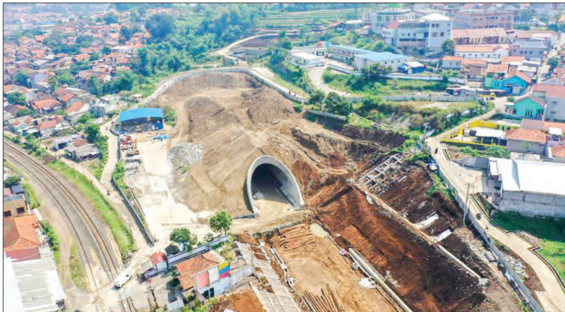
The No. 10 tunnel of the Jakarta-Bandung High Speed Railway (HSR) is seen in West Bandung Regency, West Java province, Indonesia, 6 August 2021. The No. 10 tunnel of the Jakarta-Bandung HSR in Indonesia was completed, the railway's operator said on Saturday. PHOTO: XINHUA
