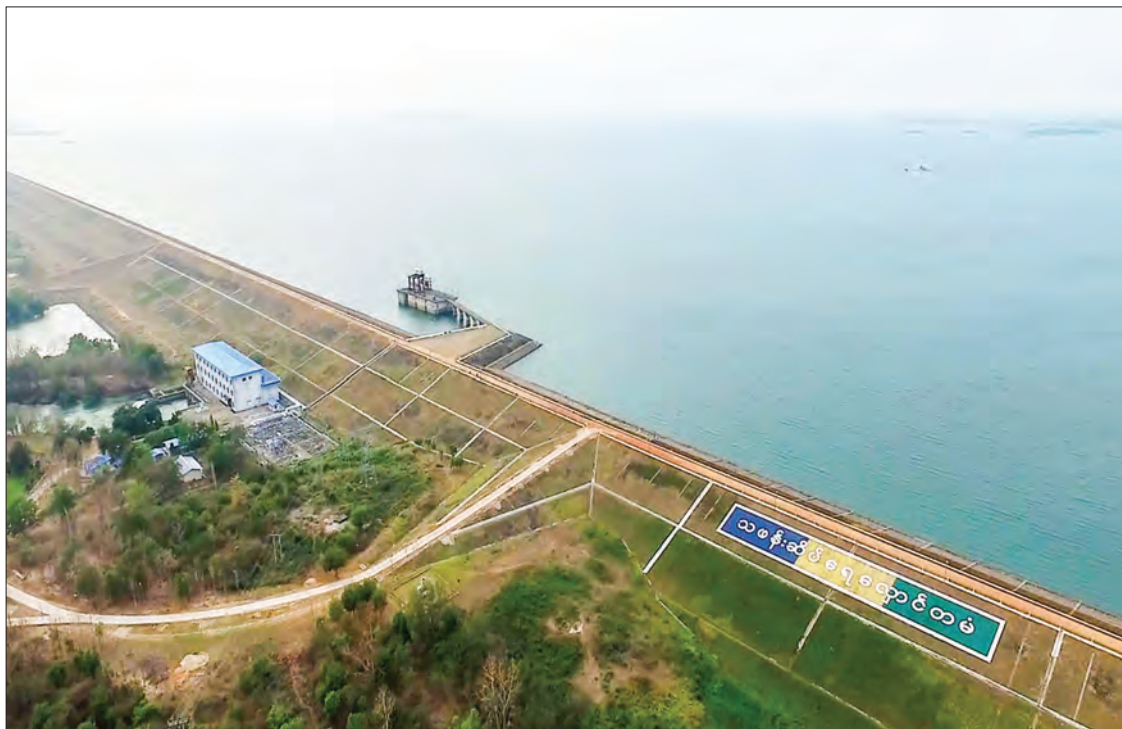
Thaphan Seik Dam is seen intact after the 6.3-magnitude earthquake whose epicentre is closest to it.
