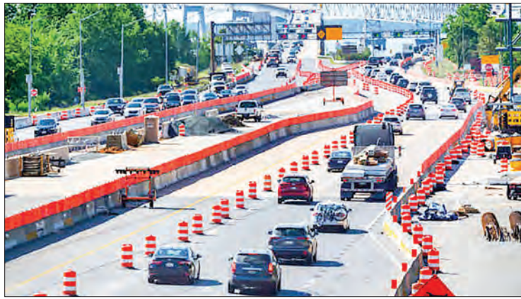
Traffic flows through a construction area near the Bay Bridge in Annapolis, Maryland on 21 May, 2021. PHOTO: JIM WATSON/ AFP
