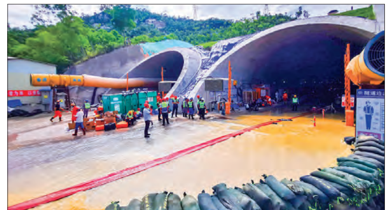
Rescuers build embankments to pump out water from a flooded tunnel in Zhuhai city in south China's Guangdong province Friday, 16 July, 2021. Divers have been dispatched in the search for 14 workers missing since water flooded a tunnel under construction in southern China three days ago, authorities said Sunday, 18 July, 2021. PHOTO: XINHUA
