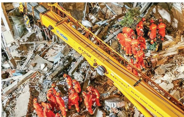
The Siji Kaiyuan hotel collapsed on Monday and no reason for the disaster has yet been given. PHOTO: CNS/AFP
