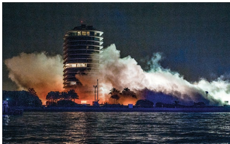
Smoke rises above as the rest of the Champlain South tower is demolished in Surfside, Florida, north of Miami Beach, late on 4 July 2021. PHOTO: AFP
