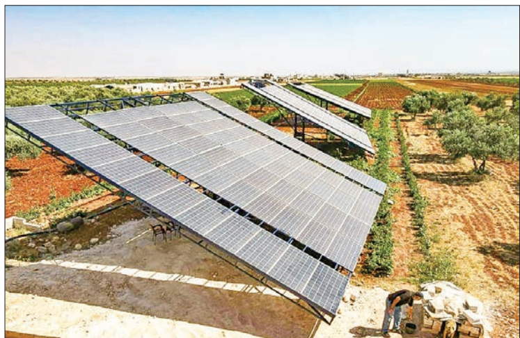
In rebel-held Syria, large solar panels have been installed to not only power homes but also for farmers, to pump water to irrigate fields.
